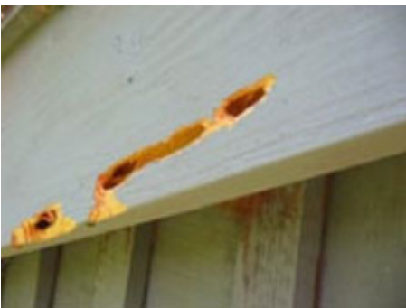
Figure 4. Carpenter bee gallery exposed in wood.
