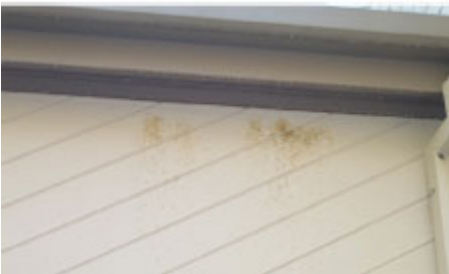
Figure 3. Carpenter bee staining on siding below the fascia.
