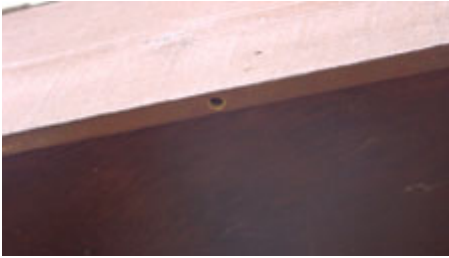
Figure 2. Carpenter bee entrance hole in fascia.
